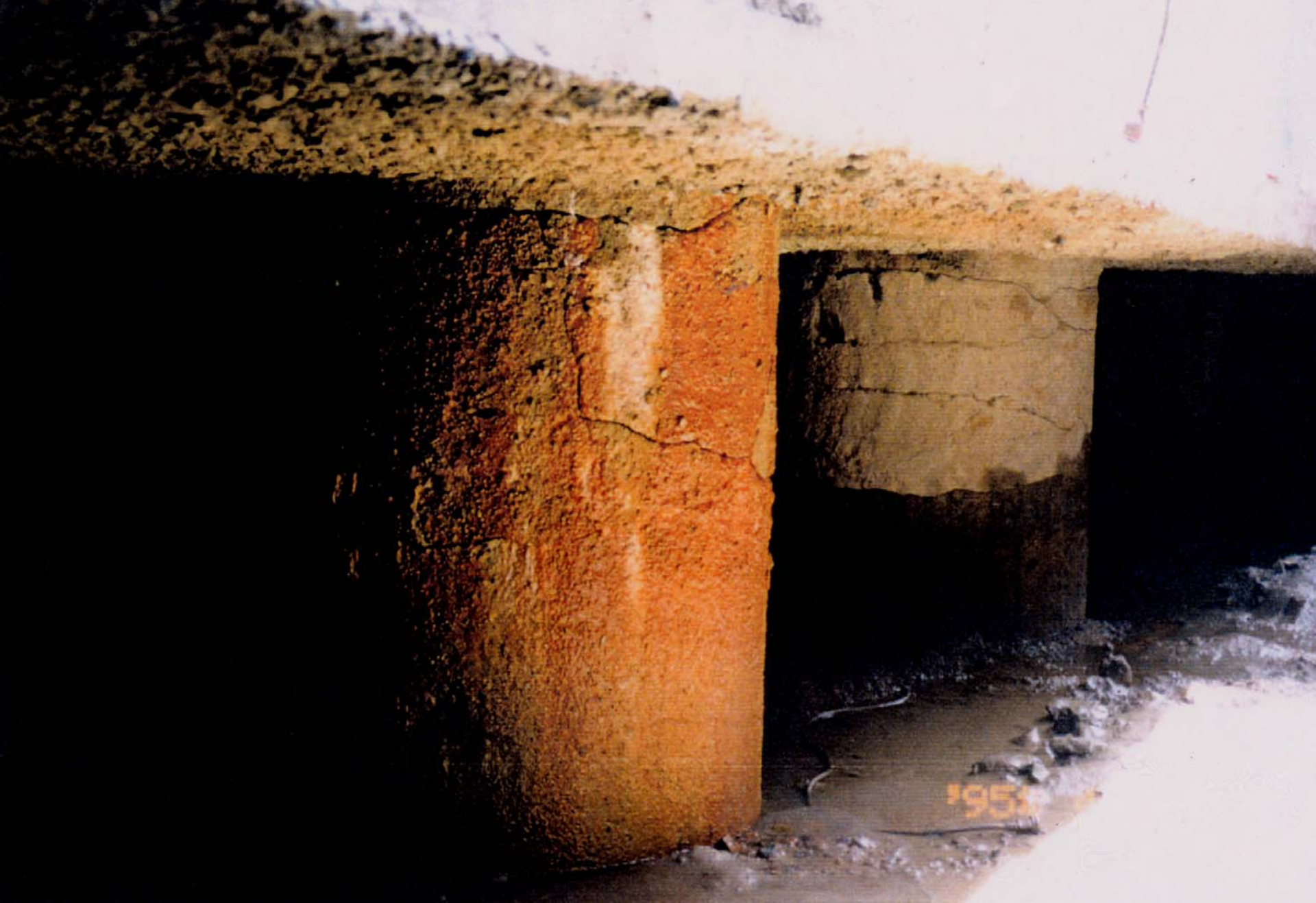
Cracks on the cast-in-place concrete pile
