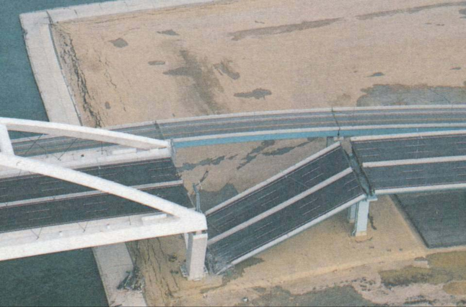
Fall down of superstructure (Nishinomiya Br.)
